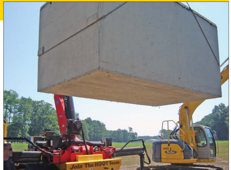
A work crew delivers a 17,000-pound Hoot H-1000 AND treatment system with 1,000 gpd capacity, built on 1,469-gallon pump tank. The unit was moved with a crane truck built by Hoot Aerobic Systems.
